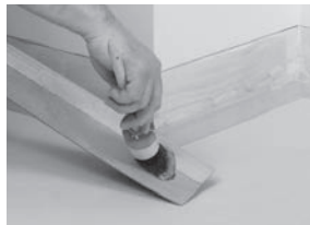
Apply glue on the floor and against the wall till the line.
